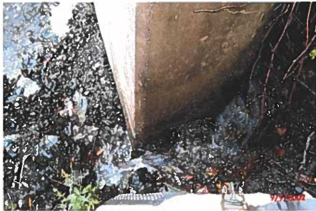
Photo 15 – Leakage at left downstream wingwall
