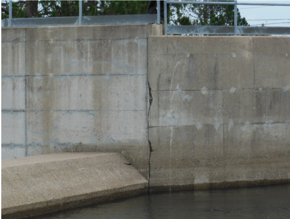
Photo 27: Spruce Lake Dam – Concrete Spillway Joint of right abutment wall and wing wall
