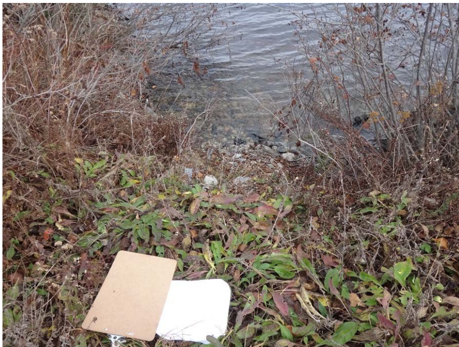
Photo 18: Menzies Lake Saddle Dyke 2 Erosion/beaching at upstream waterline
