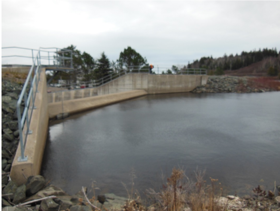
Photo 23: Spruce Lake Dam – Concrete Spillway View from upstream toe of left wingwall
