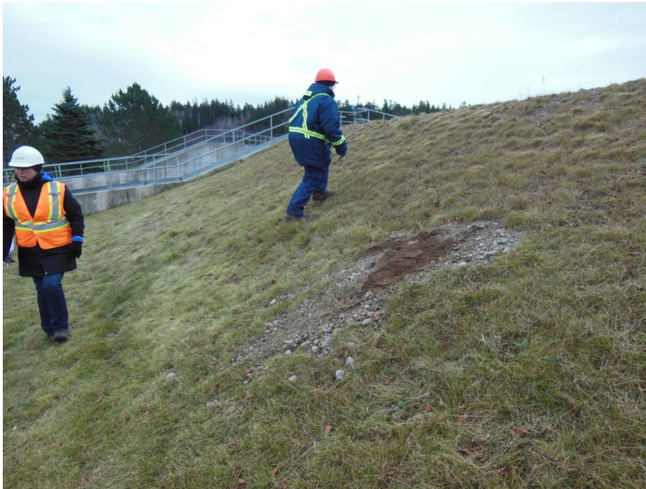
Photo 35: Spruce Lake Dam – Left Embankment Area of granular material on downstream slope (appeared to be dumped)
