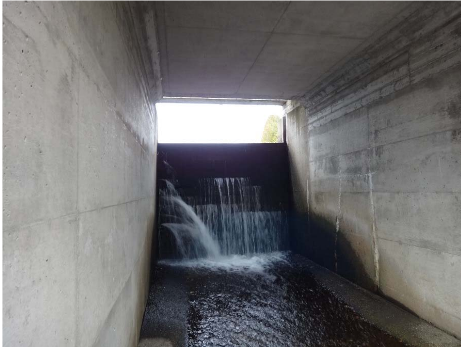
Photo 11: Menzies Lake Control Structure Leakage through stoplogs
