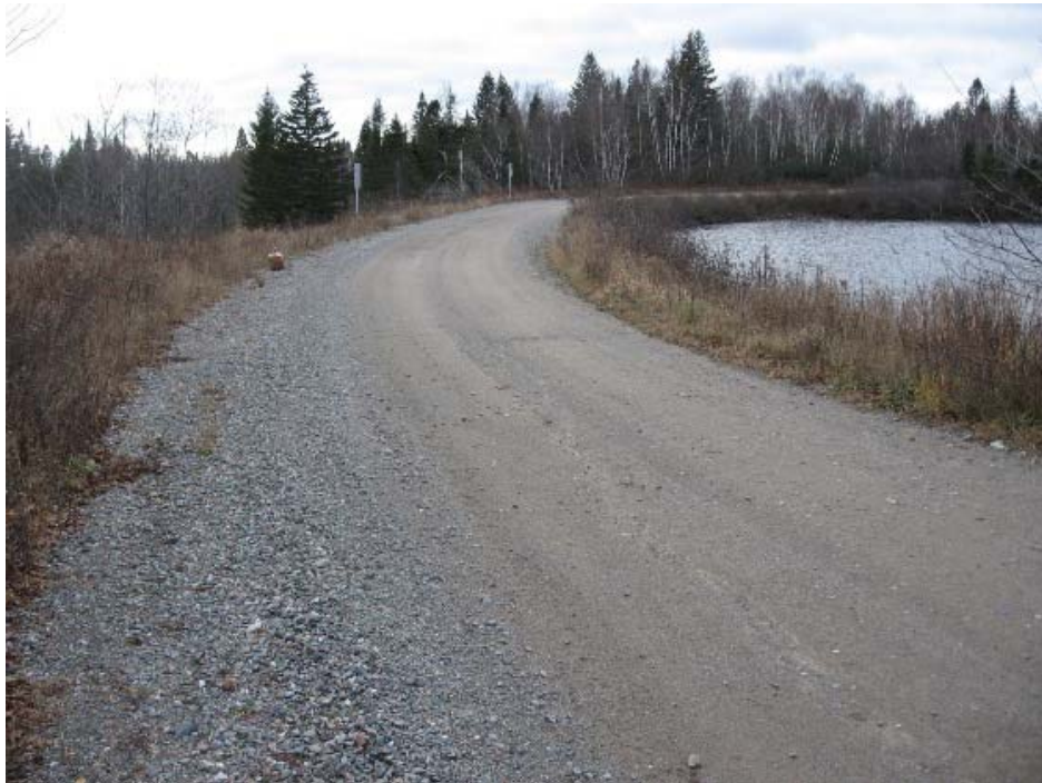
Photo 13: Menzies Lake Saddle Dyke 1 Crest of dam, from left abutment looking West
