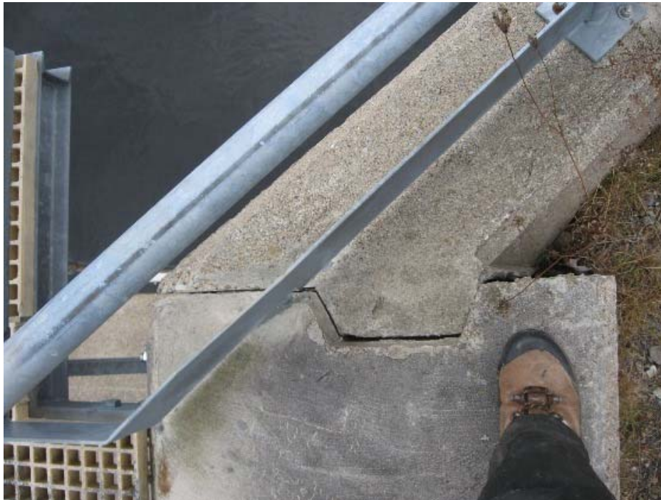
Photo 29: Spruce Lake Dam – Concrete Spillway Joint of left abutment wall and wing wall
