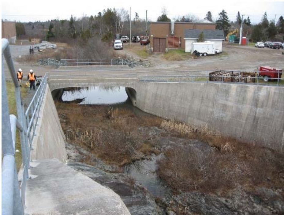
Photo 30: Spruce Lake Dam – Concrete Spillway Downstream retaining walls of discharge channel and precast concrete arch culvert
