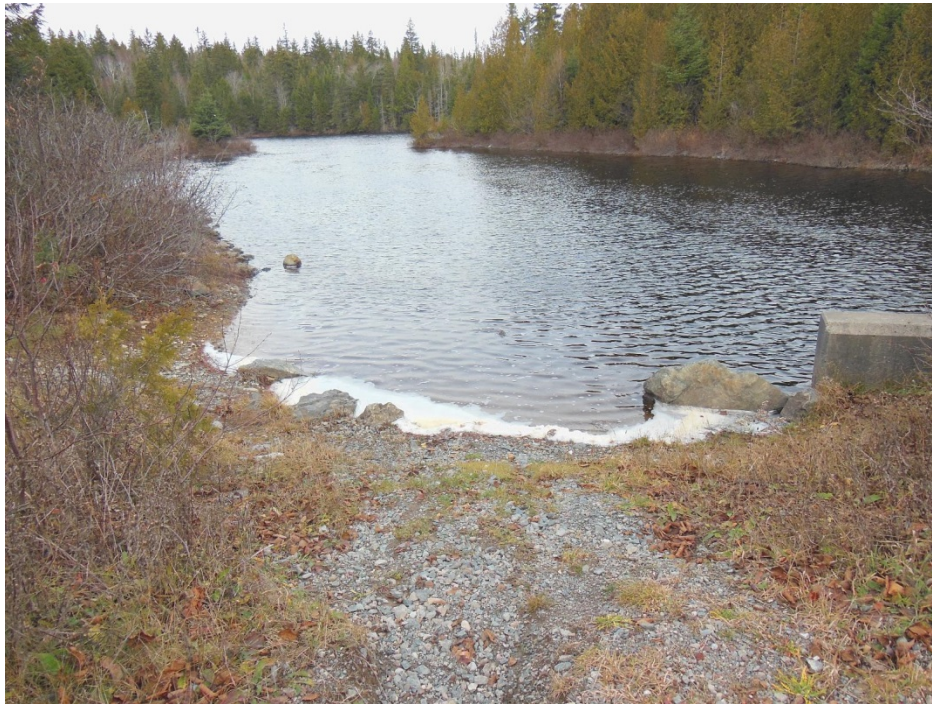
Photo 3: Menzies Lake Control Structure Looking upstream from the right abutment of the structure
