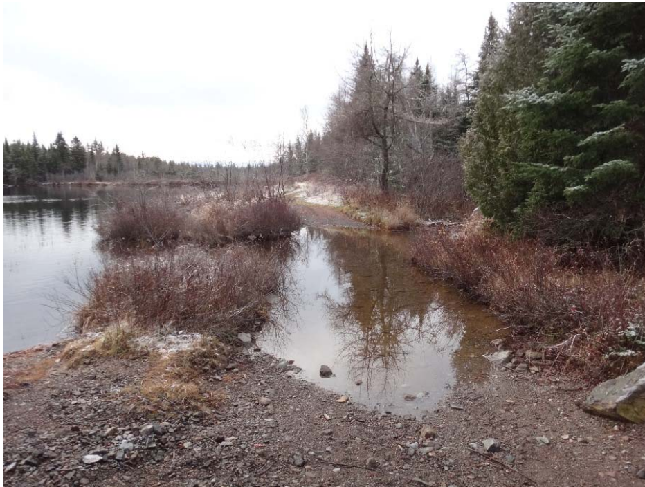
Photo 48: McBrien Southwest Dam View of breach near right abutment
