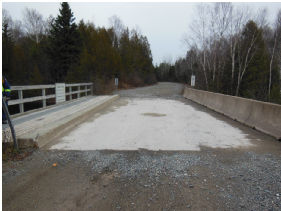
Photo 6: Menzies Lake Control Structure Looking at the crest from the right abutment of the structure
