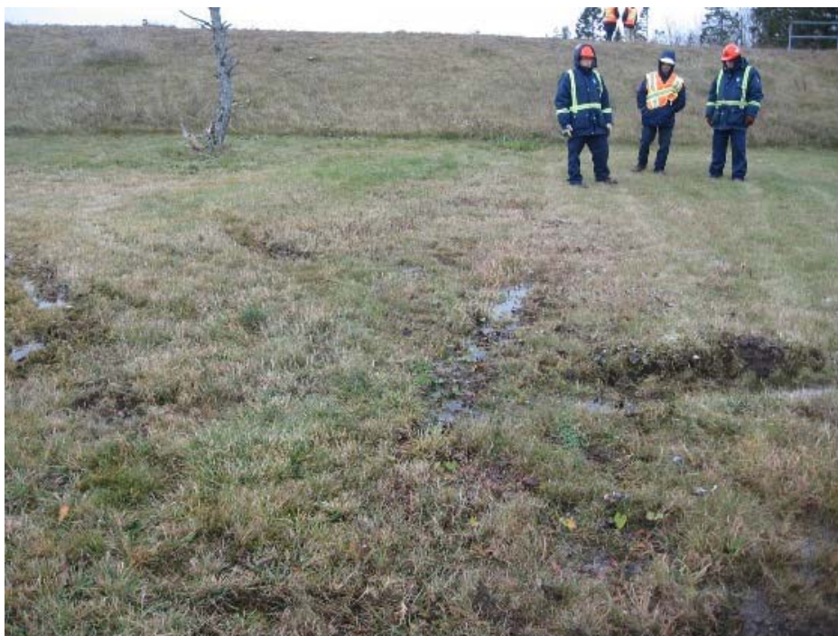
Photo 40: Spruce Lake Dam – Right Embankment Wetness (from seepage) beyond downstream toe
