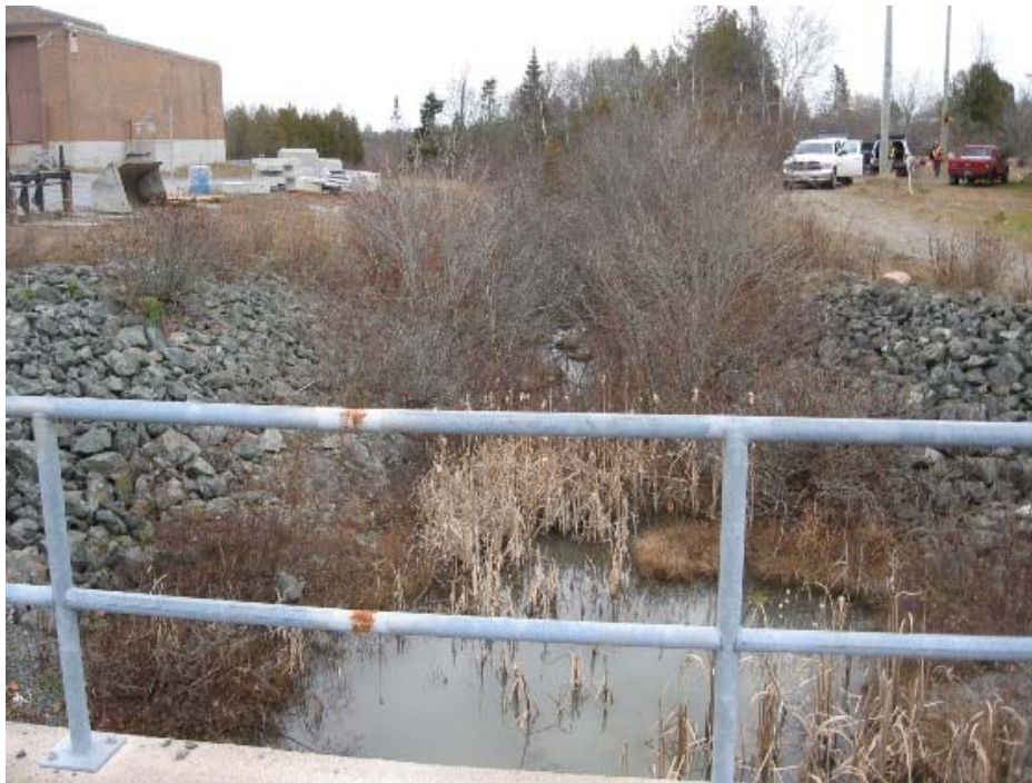
Photo 31: Spruce Lake Dam – Concrete Spillway Discharge channel downstream of precast concrete arch culvert
