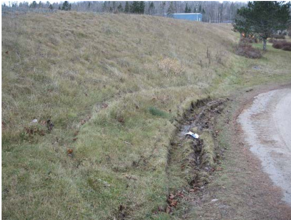
Photo 39: Spruce Lake Dam – Right Embankment Downstream slope, note thick grass and damage at downstream toe
