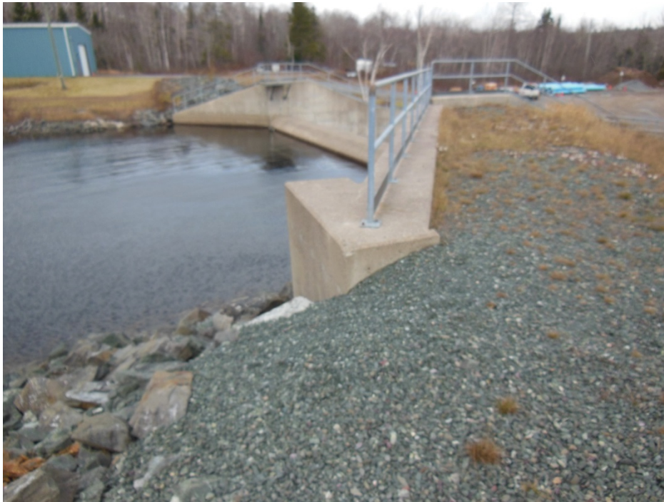
Photo 41: Spruce Lake Dam – Right Embankment Crest material migrating into riprap at abutment of spillway wing wall
