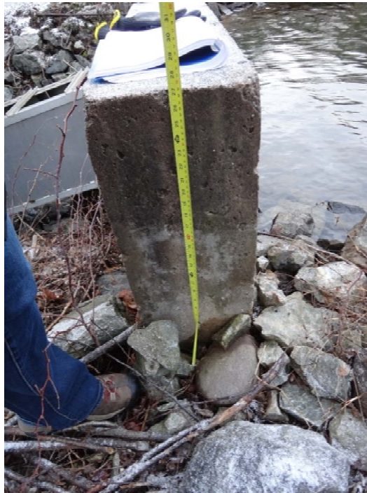
Photo 46: Hunter Lake Dam Left abutment, corewall is not backfilled and water can go around the dam
