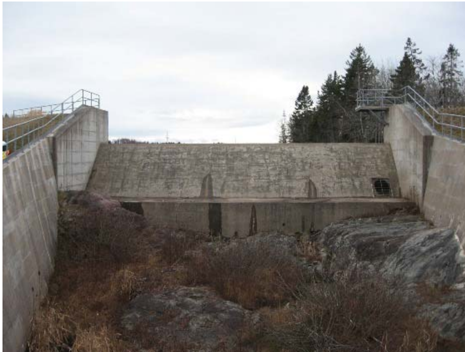
Photo 25: Spruce Lake Dam – Concrete Spillway Downstream face of spillway structure and retaining walls
