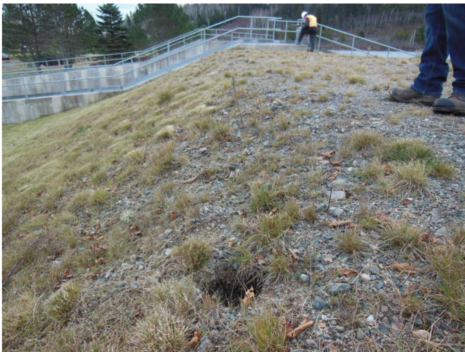
Photo 34: Spruce Lake Dam – Left Embankment Animal hole on downstream slope near crest
