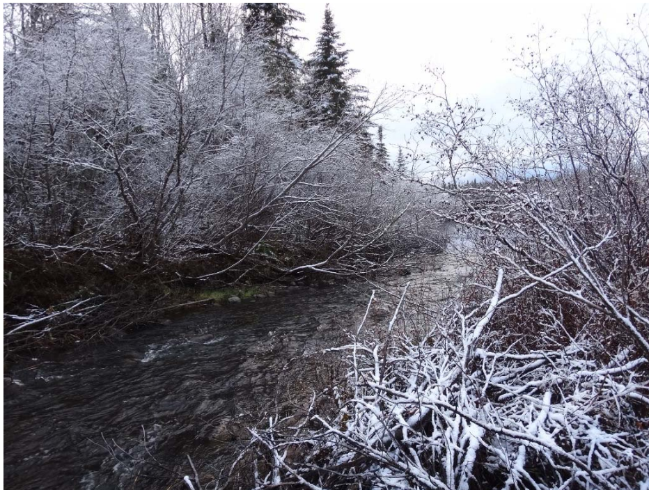
Photo 65: Otter Lake Dam Breach at Otter Lake Dam
