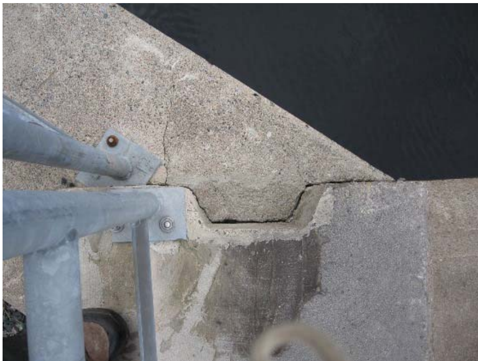
Photo 28: Spruce Lake Dam – Concrete Spillway Joint of right abutment wall and wing wall
