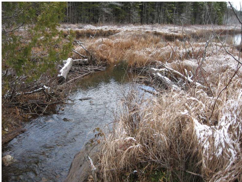
Photo 59: Terreo Lake Dam Looking downstream at breached area
