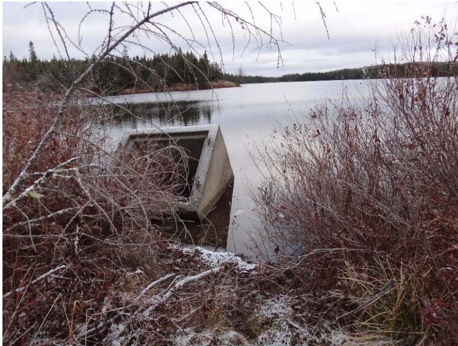
Photo 50: McBrien Southwest Dam Displaced decant structure
