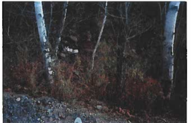
Photo 6 – Saddle Dyke 1 – Seepage at left abutment toe and trees on slope.
