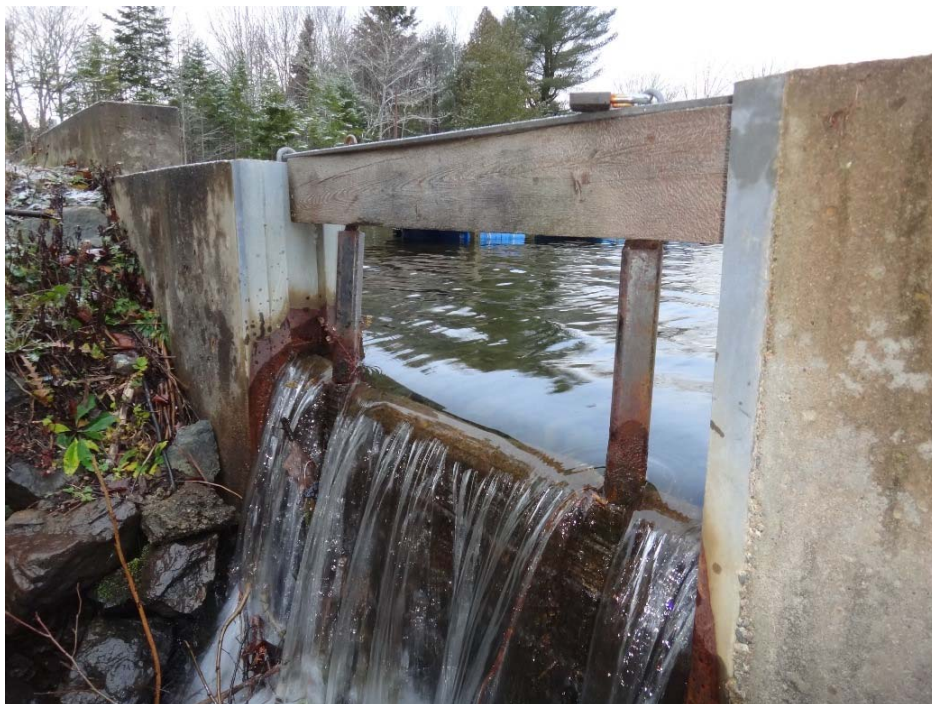
Photo 45: Hunter Lake Dam Stoplogs in place to 0.52 m below top of spillway
