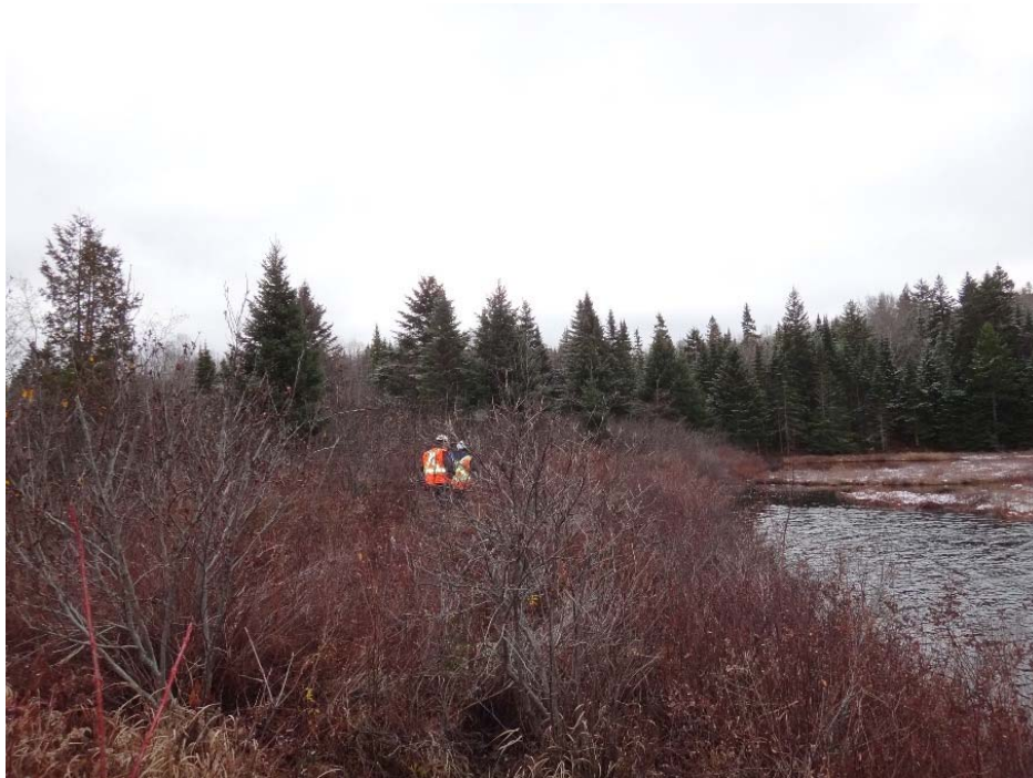
Photo 54: McBrien Southeast Dam Trees and vegetative growth on crest and upstream slope
