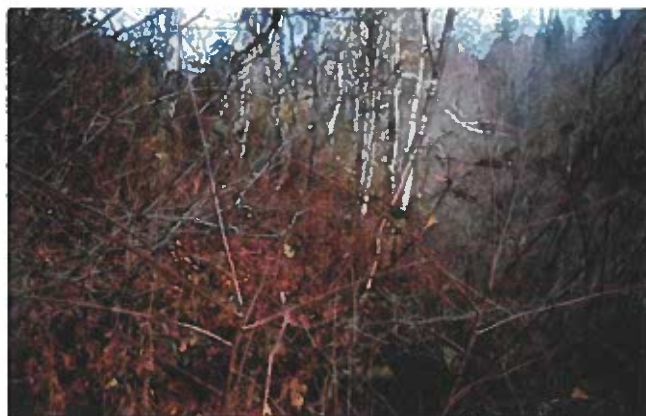
Photo 8 – Saddle Dyke 1 – tree growth on slope
