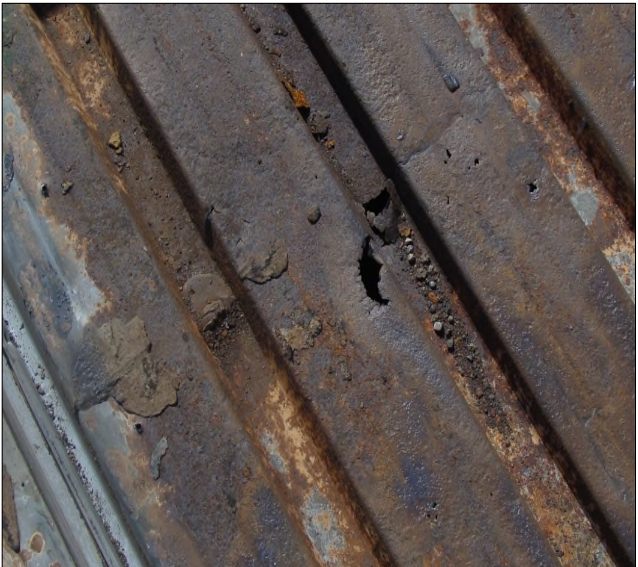
Photo of Level 4: Severe Corrosion With Holes
