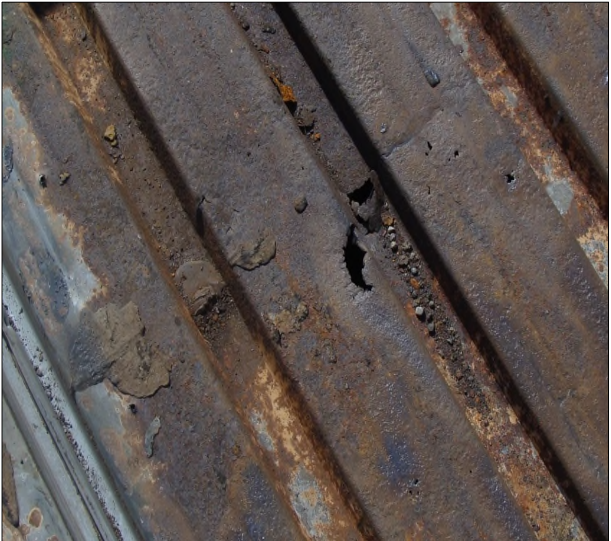
Photo of Level 4: Severe Corrosion With Holes
