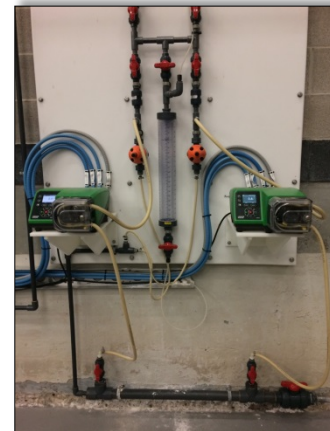
Figure 3.7.2-1: Temporary Orthophosphate Dosing System - Spruce Lake WTP
