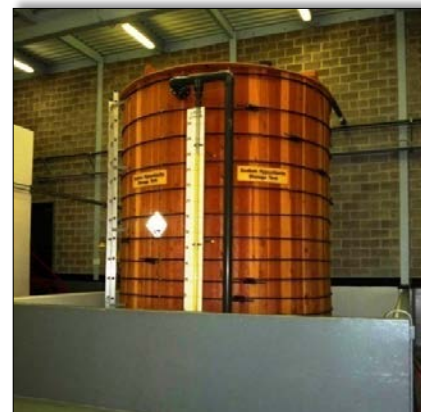
Figure 3.7.1-1: Sodium Hypochlorite Storage Tank - Spruce Lake WTP
