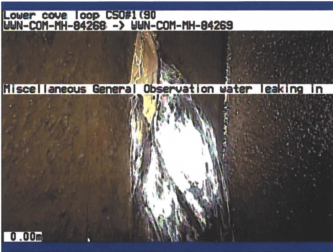
Figure 7: Visible infiltration to the left of the flap gate of CSO No. 1
