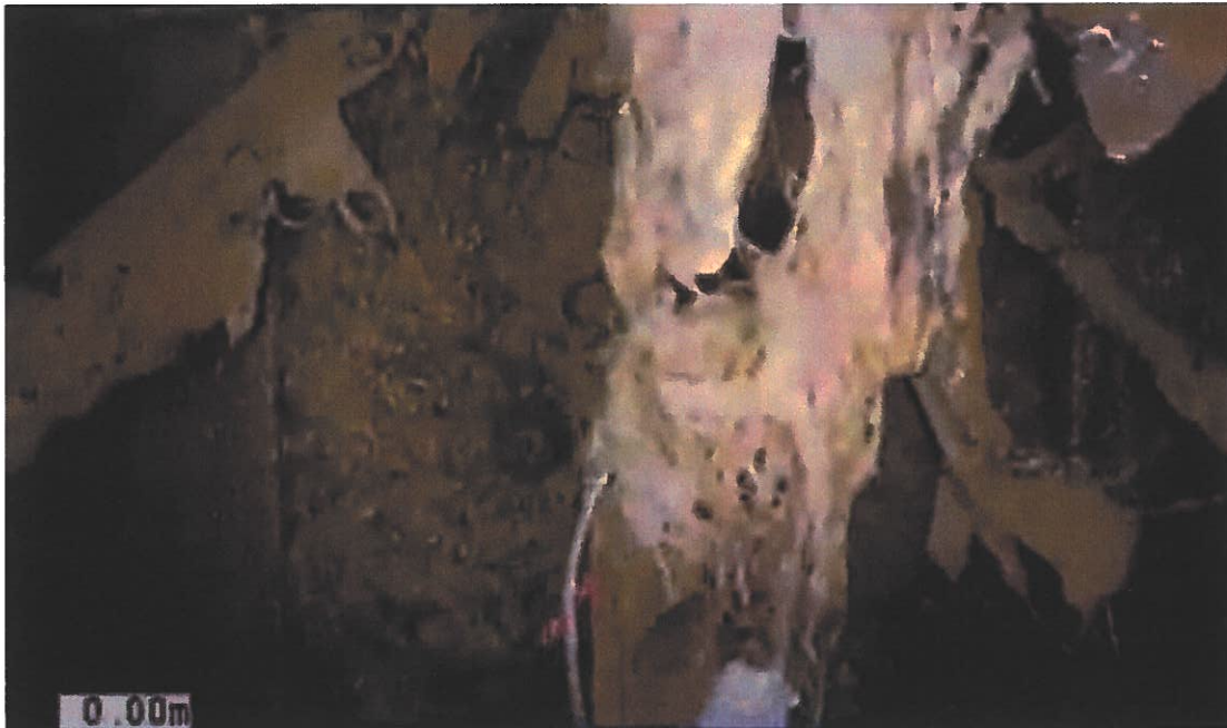
Figure 3: Concrete cut-out below the flap gate downstream of CSO No. 1, including segregated grout (2:20 of video CSO#1 (90 Manhole WVN-COM-MH-84269.mp4))
