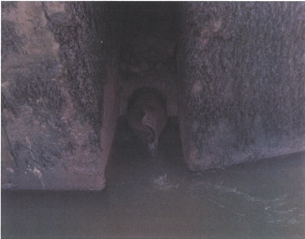
Figure 2: Damaged Tideflex at Outfall
