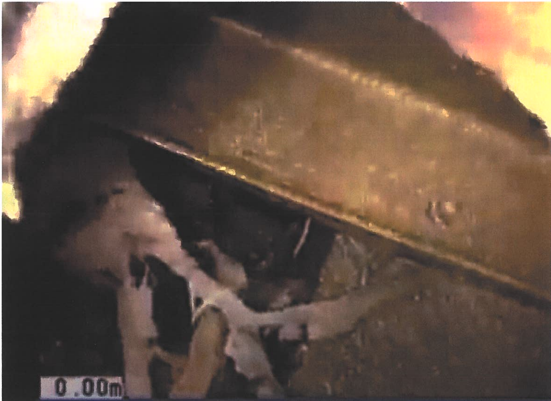
Figure 2: Concrete cut-out below the flap gate downstream of CSO No. 1, including segregated grout (1:53 of video CSO#1 (90 Manhole WWN-COM-MH-84269.mp4))
