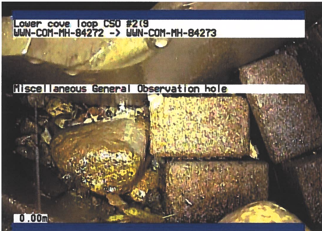
Figure 14: Perimeter of CSO No. 2's outlet pipe filled with brick and rocks. Mortar seems to be washed away
