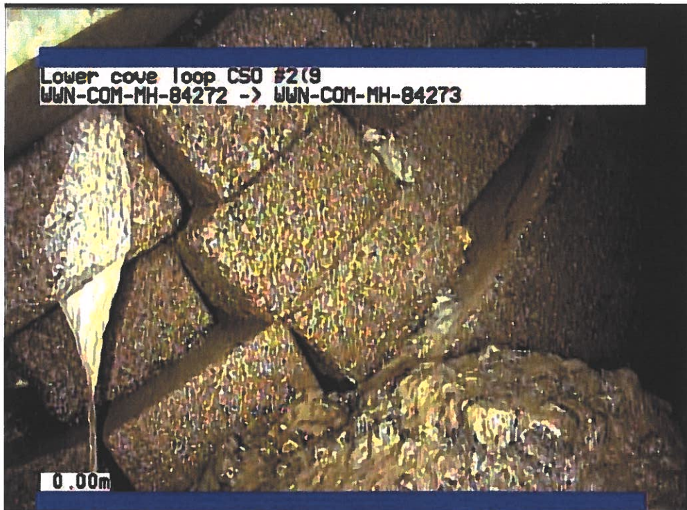
Figure 15: Perimeter of CSO No.2's outlet pipe filled with brick and rocks. Mortar seems to be washed away
