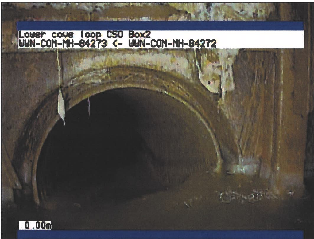
Figure 20: Debris accumulated on the bottom lip of the sluice gate on the upstream side of CSO No, 2
