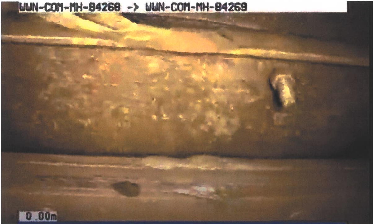
Figure 5: Sealant around flap gate in CSO No. 1 dislodged and no longer sealing (90 Manhole WUN-COM-MH-84269.mp4)
