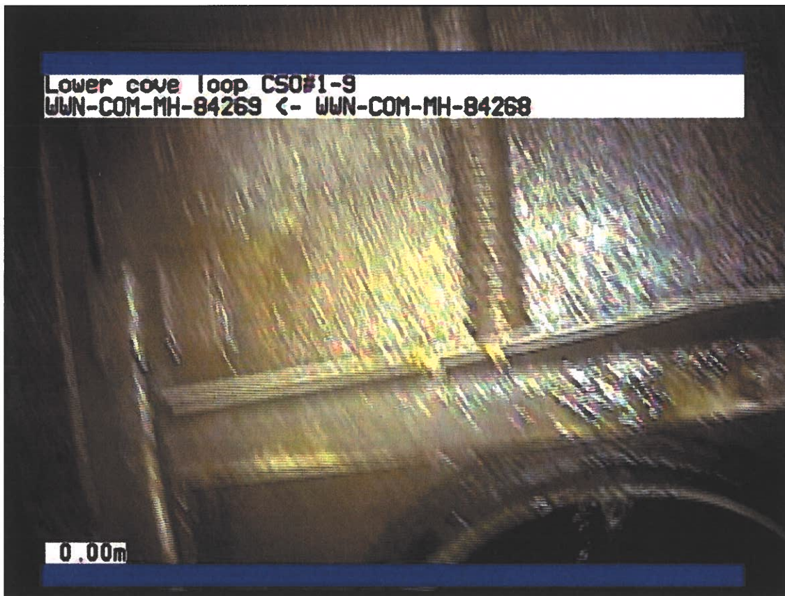
Figure 12: Sluice gate of CSO No.1's outlet pipe is visibly bent
