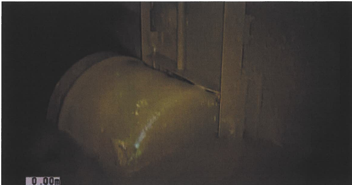
Figure 11: 450 mm diameter PVC cap blocking the sluice gate and outlet pipe of CSO No. 1
