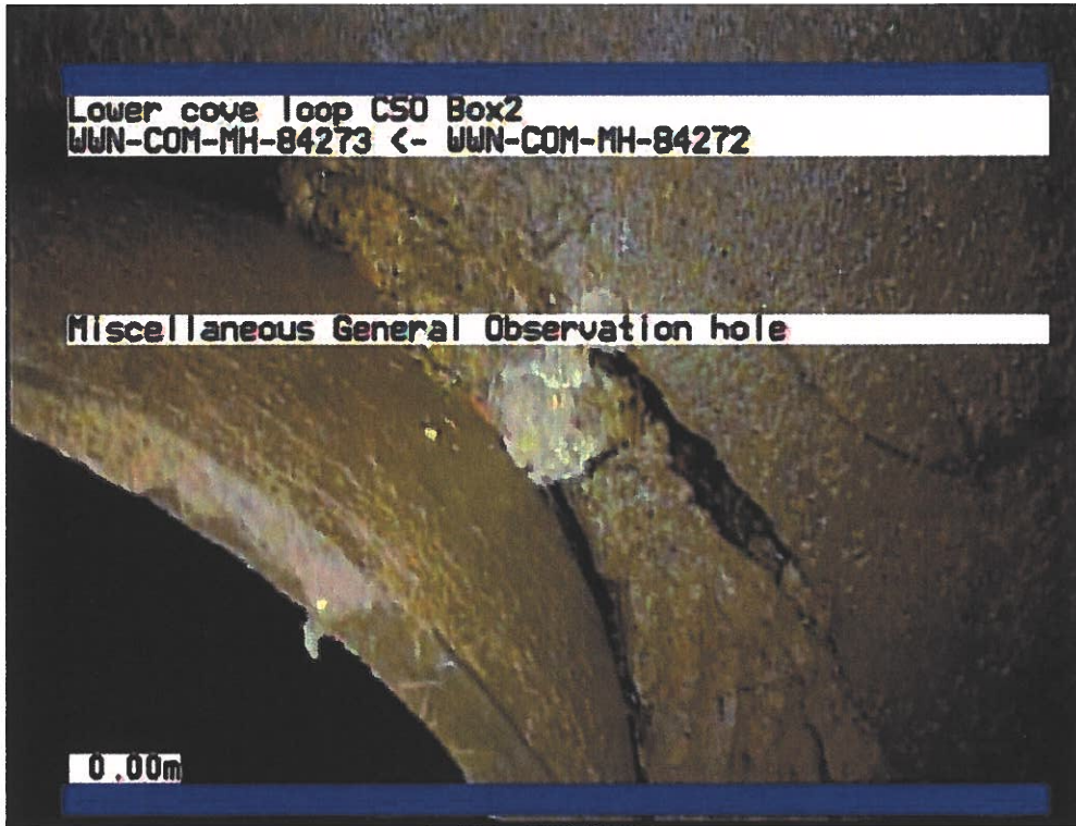
Figure 17: Perimeter of CSO No.2's inlet pipe filled with brick and rocks. Mortar seems to be washed away
