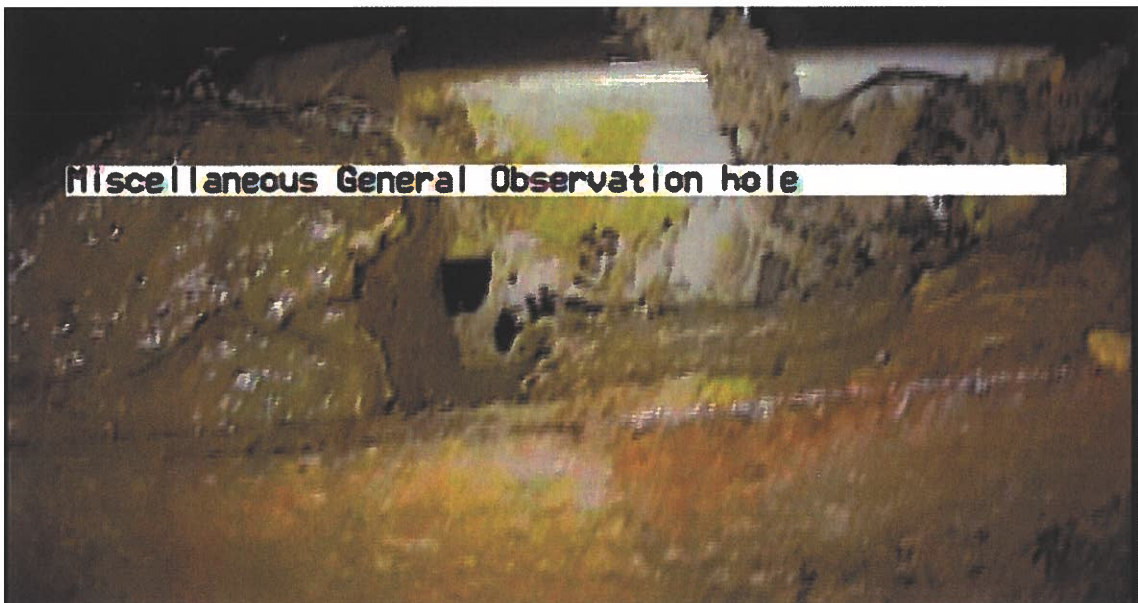
Figure 10: Top metal plate blocking the cut-out concrete below the flap gate on the upstream side of CSO No. 1. Visible gap between the flap gate and the concrete/grout.
