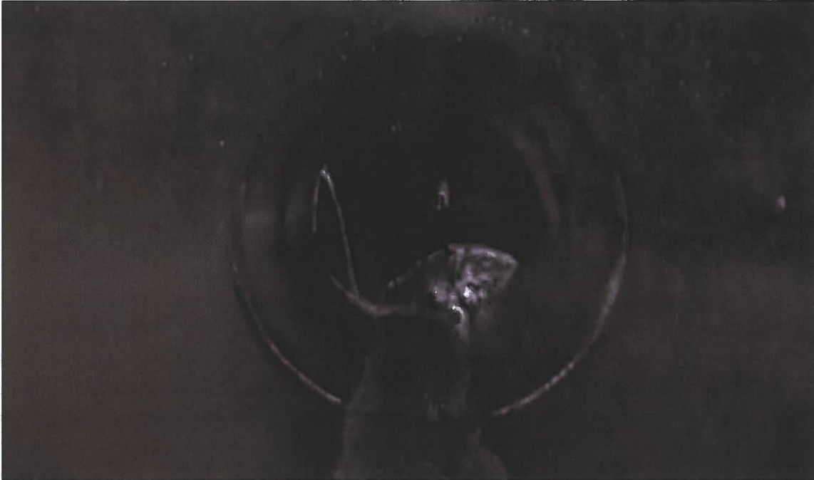
Figure 1: Infiltration inside of CSO No. 1's overflow pipe (0:19 of video CSO#1 (90 Manhole WWN-COM-MH-84269.mp4))
