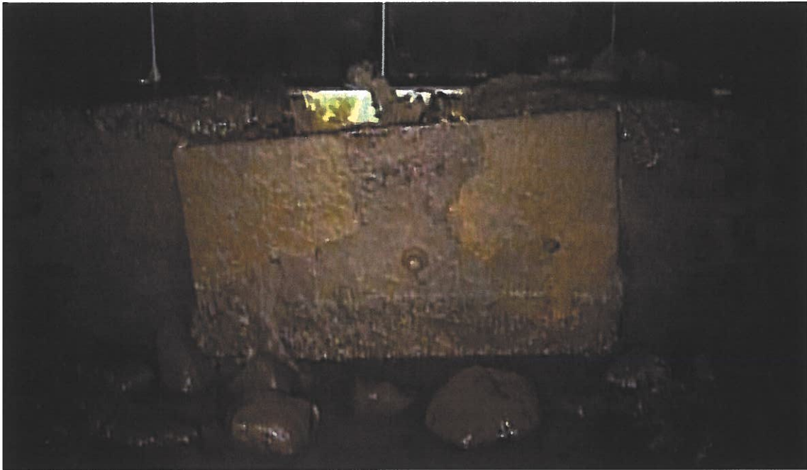
Figure 9: Metal plate blocking the cut-out concrete below the flap gate on the upstream side of CSO No. 1
