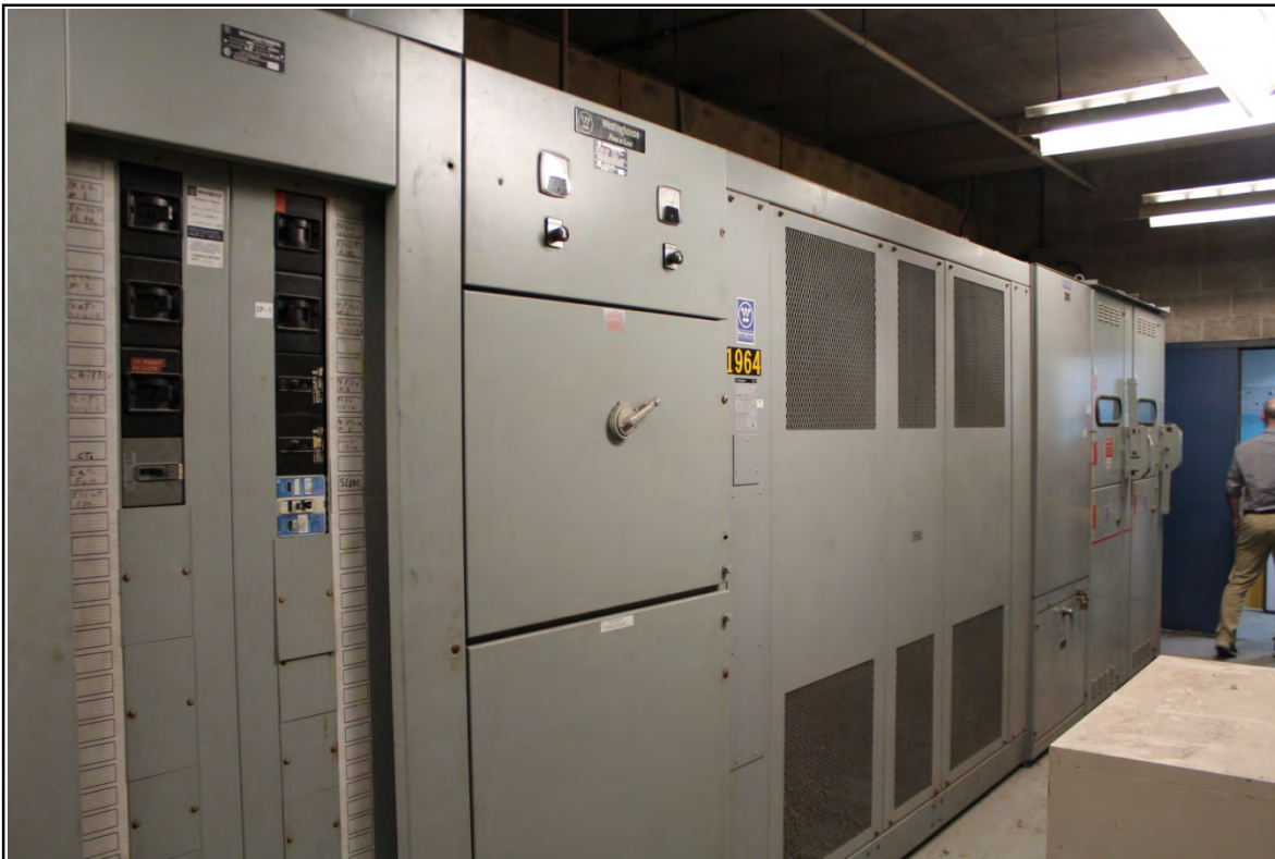
Photo 30: Main Power Supply
