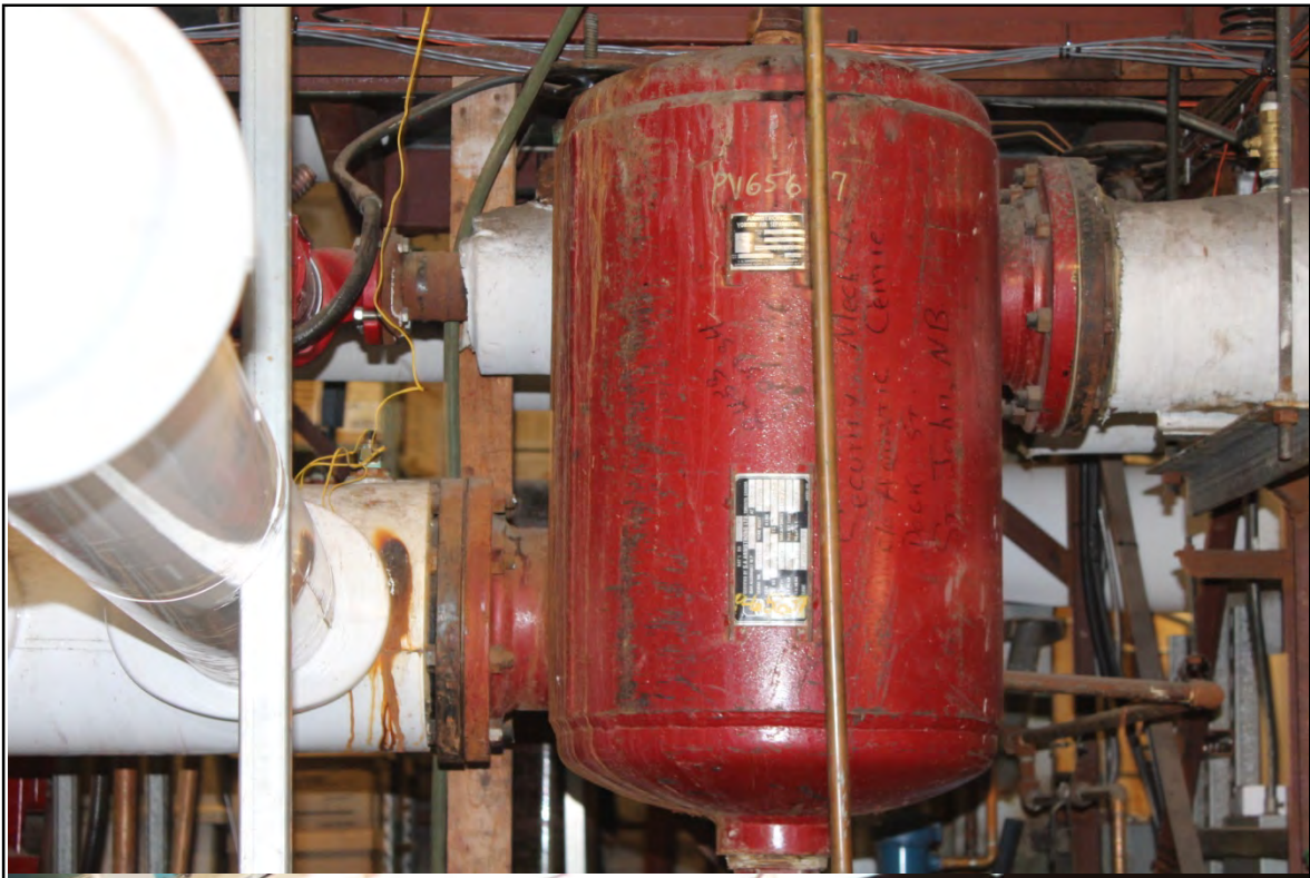
Photo 24: Vortex Air Separator
