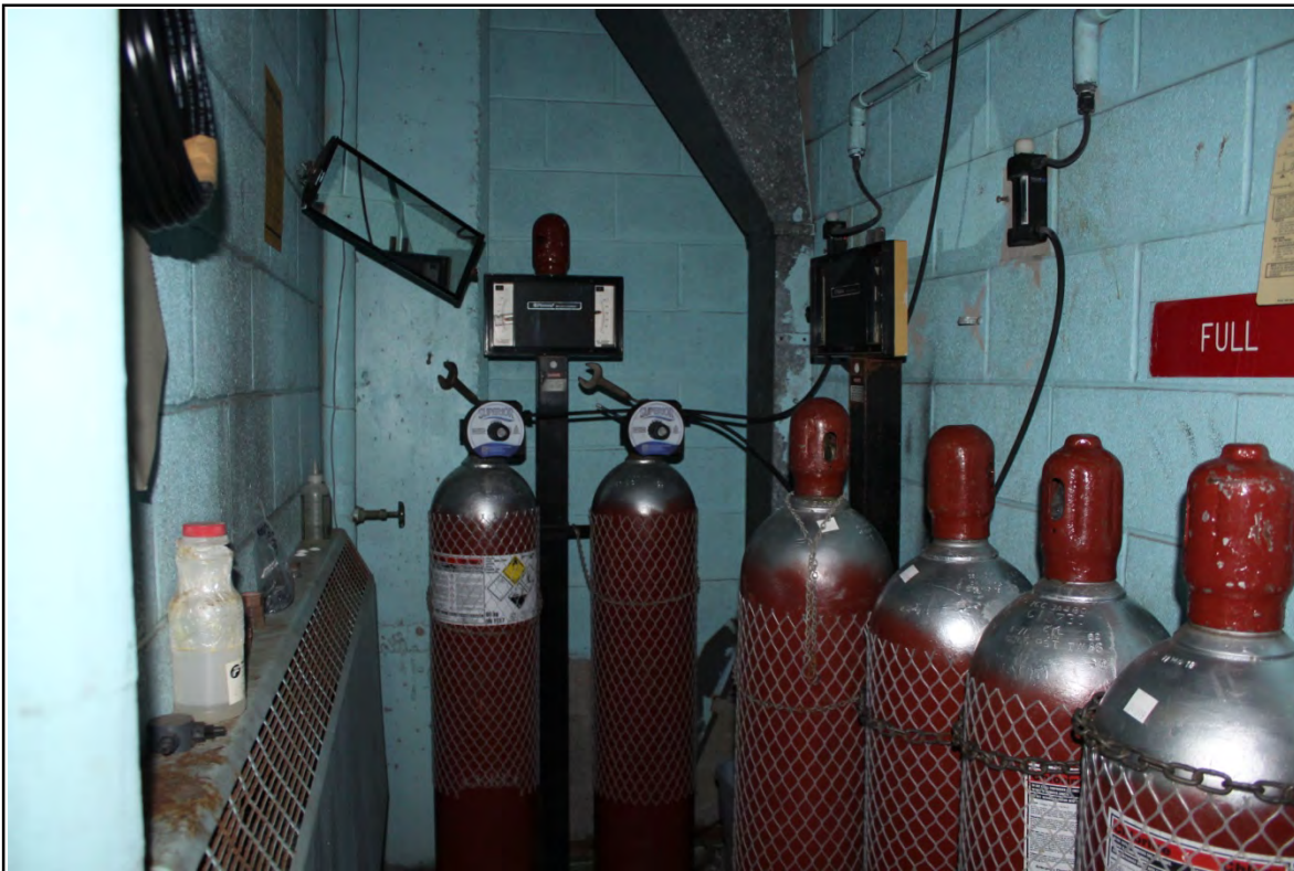
Photo 26: Chlorine Tanks And Detectors/Gauges
