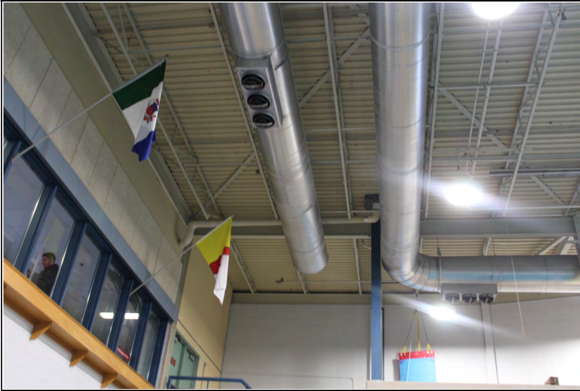
Photo 25: Swimming Pool Ventilation System
