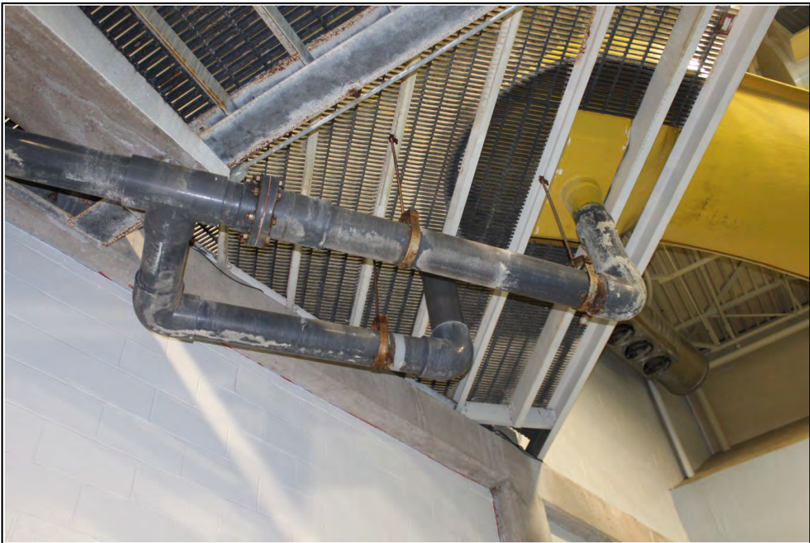
Photo 18: Corrosion And Rust On Piping And Hanging Pipe Clamps
