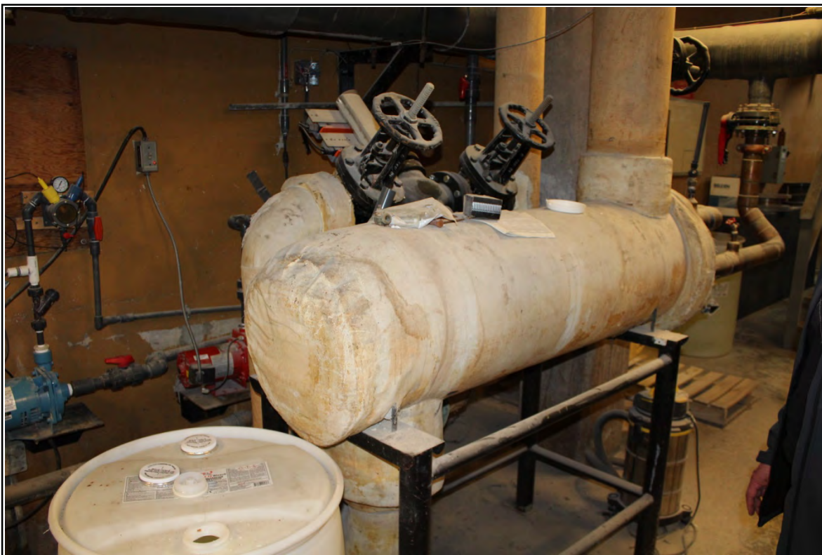
Photo 22: Shell And Tube Heat Exchanger (Main Pool)
