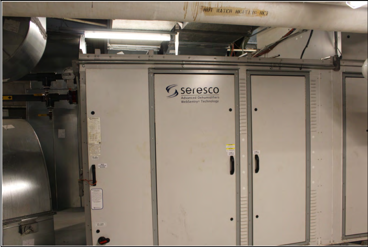
Photo 23: Facilities Dehumidifier System
