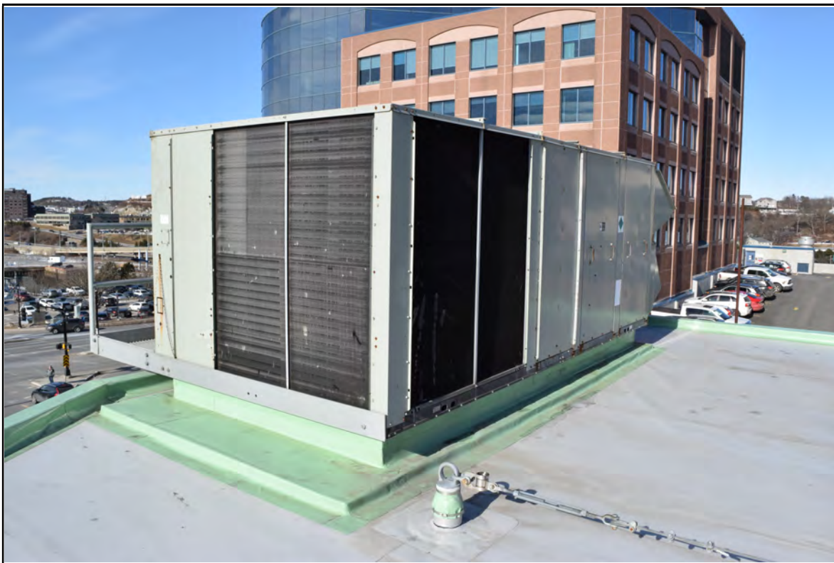
Photo 10: Trane Rooftop Unit
