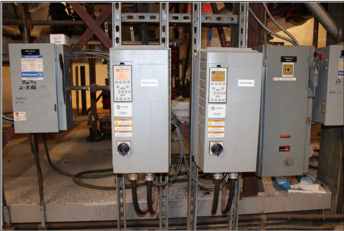
Photo 28: Variable Frequency Drives
