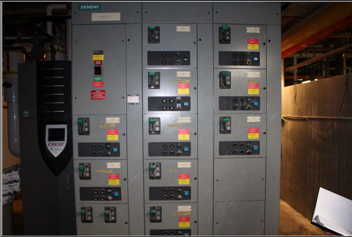
Photo 29: Motor Control Center
